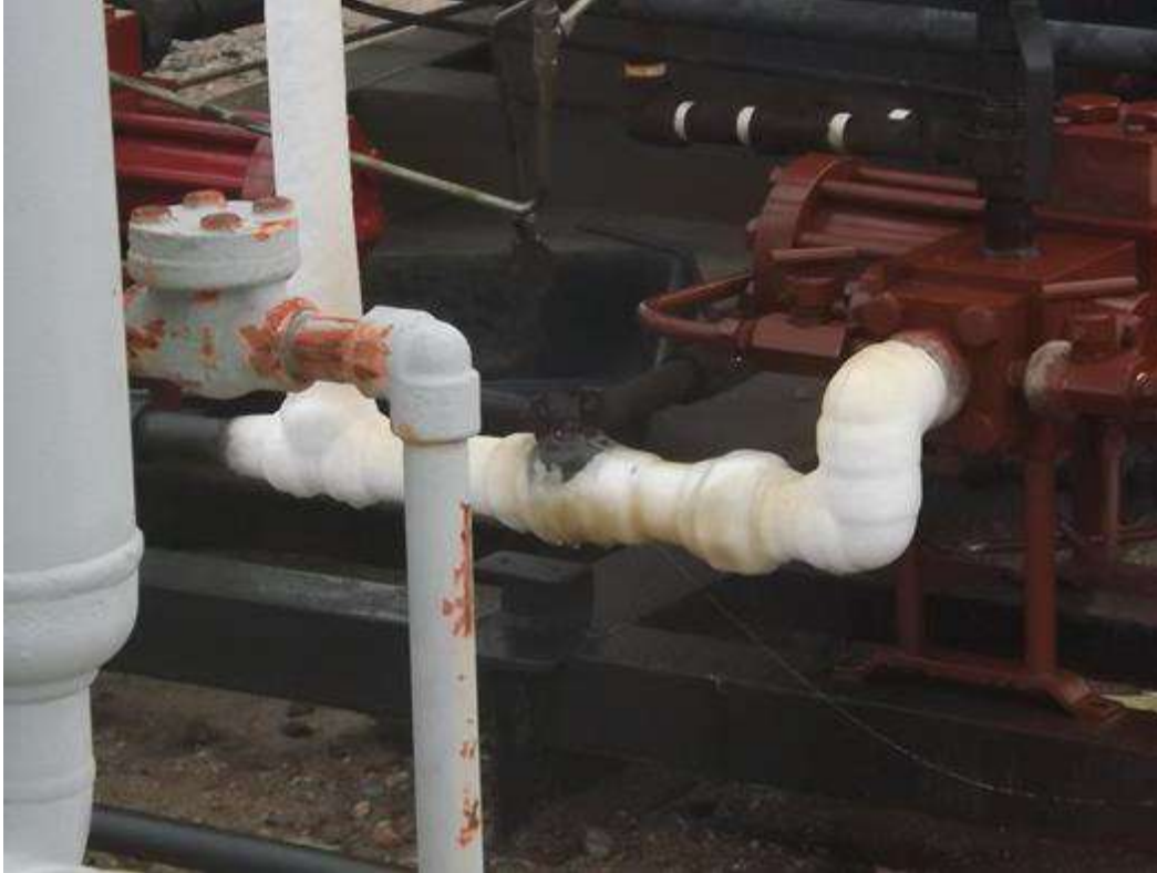
Figure S4. Photograph of the wet glycol discharge piping where the emission source was identified. The equipment was determined to be a Kimray 21020 PV model glycol pump. The maximum emission rate from the event was determined through interaction with the pump manufacturer and parameters recorded on-site.
